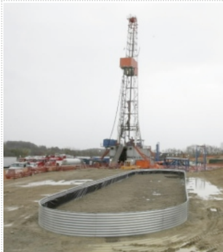
The drilling rig for a natural gas well into the Marcellus Shale is seen behind a foundation for equipment that remains on site after the well is tapped in Houston, Pa., in 2008. (File photo)
